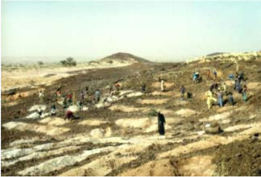
Photo 8: Erosion protection carried out by the villagers as part of the implementation of a land use plan (Niger).
